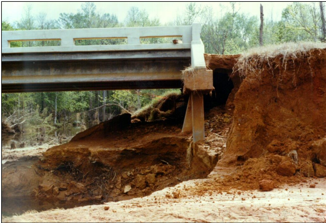
Figure 3.2 Scour at bridge approach (Source: USGS)
